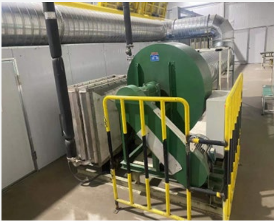
Heat Recovery Retrofit for Air Compressors
