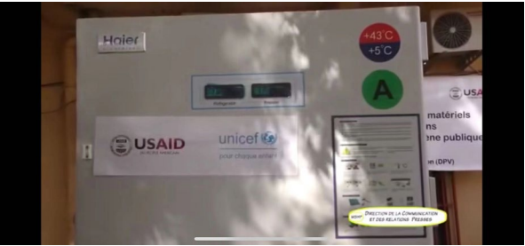
Solar-powered vaccine refrigerator installed in Burkina Faso
